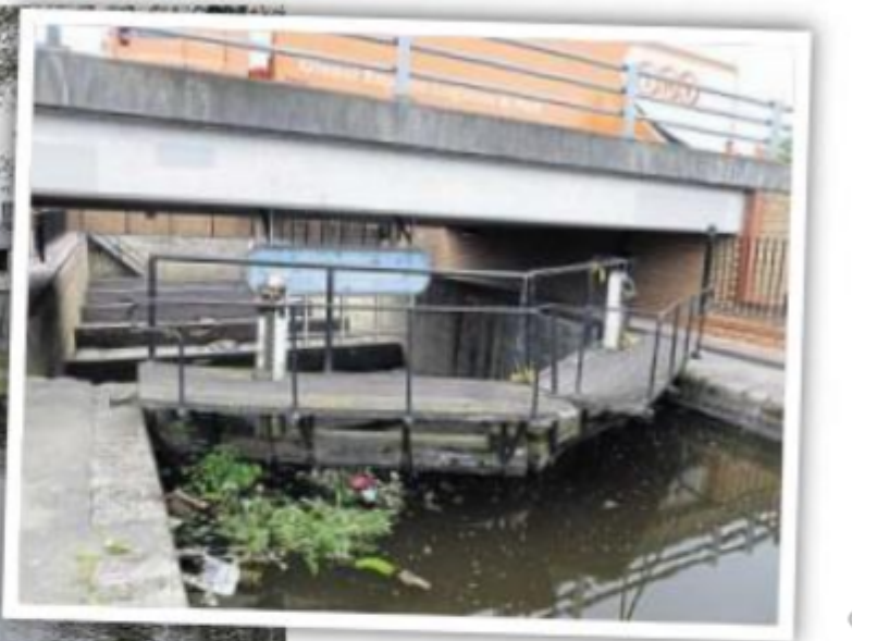
The site of the former Bull's Bridge maintenance depot as it is today. In the late 1980s the land, then in a state of semi dereliction was sold off by the British Waterways Board to Tesco to make a large supermarket and the slipways filled in to make a car park. As a token heritage-gesture the dry dock was saved, but does not operate. PHOTOS: TIM COGHLAN
